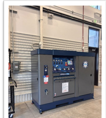
Photo of new SCBA Compressor bought by CMC.
